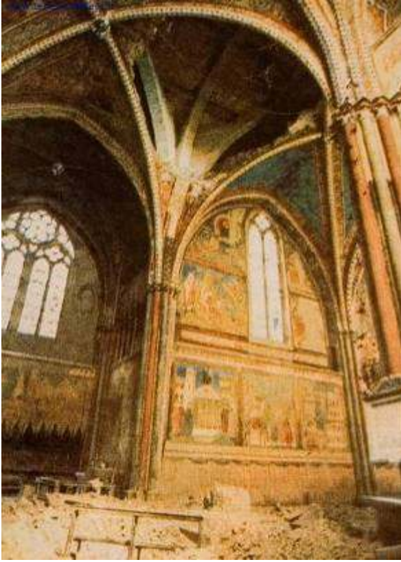
Figure 1.25. Damage cause to the upper basilica of the Franciscan complex in Assisi, due to the Umbria and Marche earthquake in 1997.
